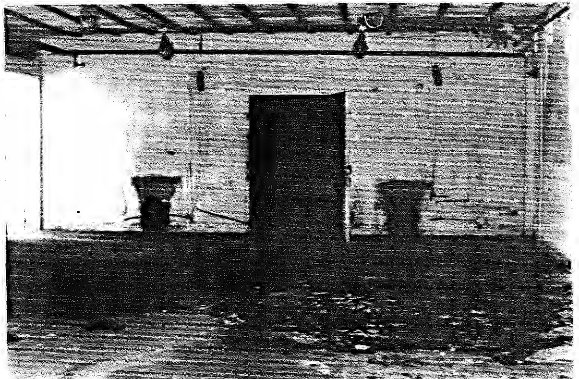
Photo 45: SEAD-16, 9/13/90. Interior of the Abandoned Deactivation Furnace - Building S-311, the doorway on the south wall is the entrance to the furnace room.
