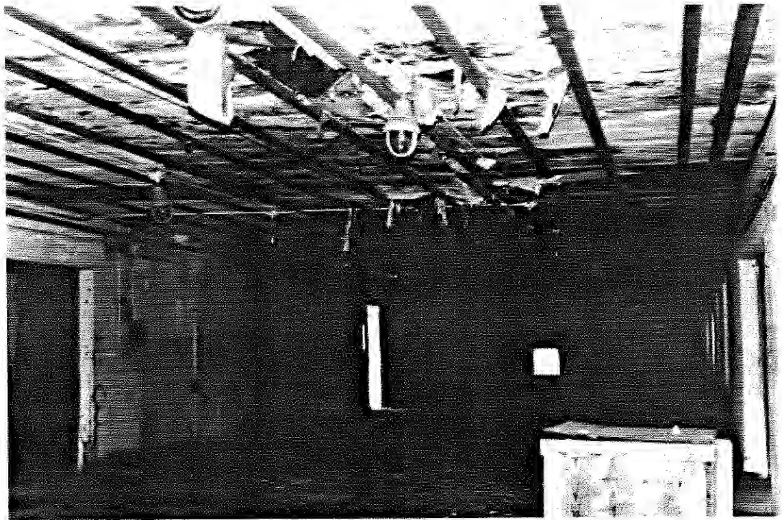
Photo 47: SEAD-16, 9/13/90. Interior of the Abandoned Deactivation Furnace - Building S-311, facing north away from the furnace room.
