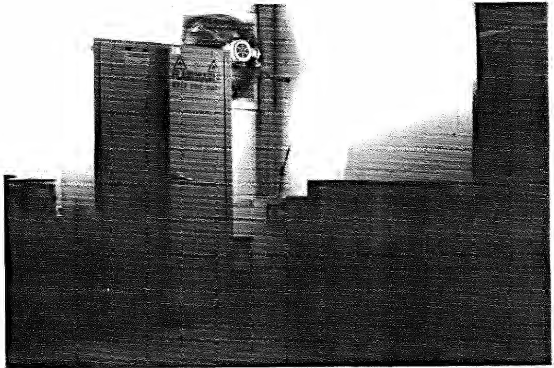
Photo 138: SEAD-56, 11/28/90. View of the Pesticide Storage Room, Herbicide and Pesticide Storage Area - Building 606, facing south.
