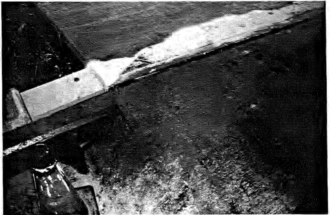
Photo 2: SEAD-1, 11/27/90. View of the monolithic concrete slab floor and 6-inch curb - Building 307, facing south.
