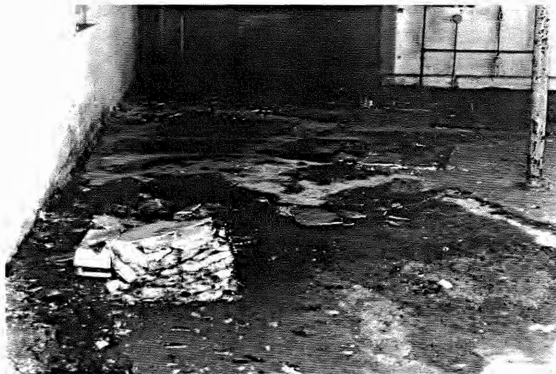
Photo 49: SEAD-16, 9/13/90. Interior of the Abandoned Deactivation Furnace - Building S-311, facing south, (view of the room adjacent to the furnace room).
