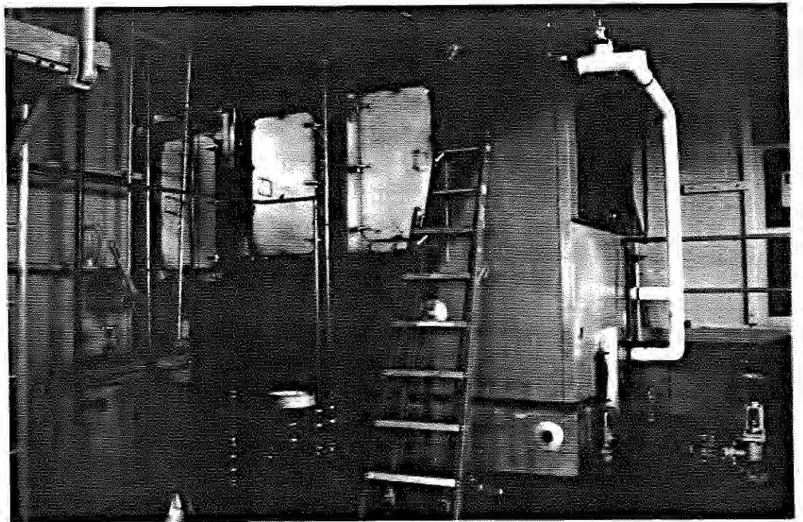
Photo 104: SEAD-37, 9/12/90. View of Waste Oil - Burning Boiler - Building 319, facing west.
