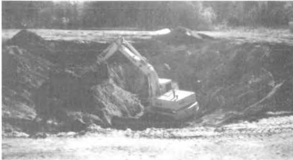
The U.S. Army Corps of Engineers excavates contaminated soil from the baseball field at the former Raritan Arsenal.
