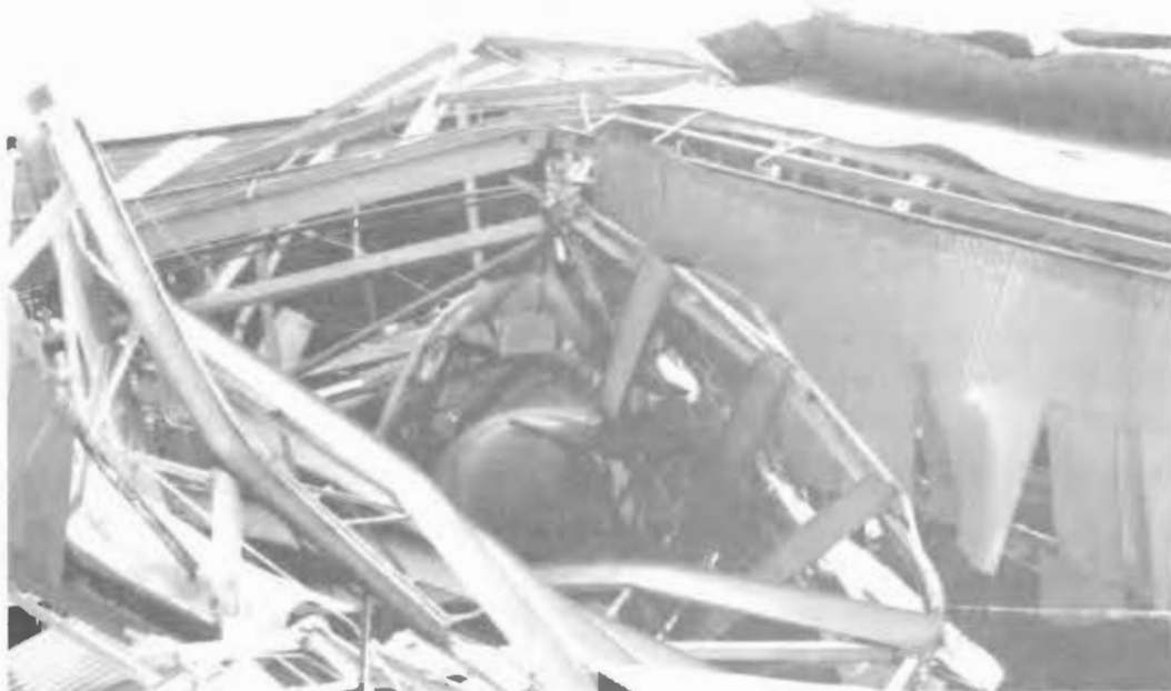
Hurricane Andrew destroyed this hangar at Homestead AFB and rendered 97 percent of installation facilities inoperable.
