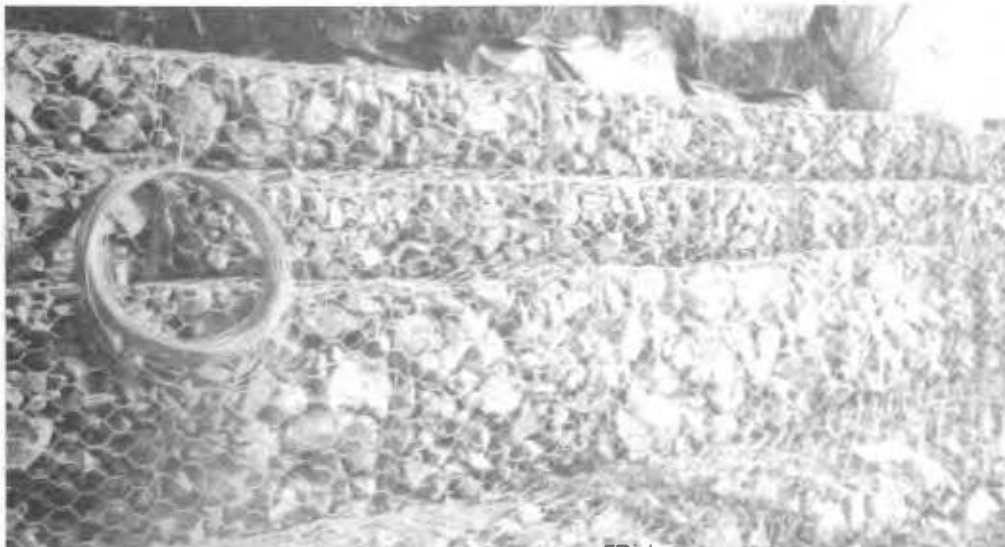
Gabion baskets were installed by the Navy along the Schuylkill River to stabilize the Girard Point Landfill at Philadelphia Naval Shipyard.
