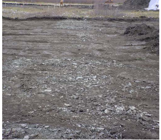
2.) AREA 1 – EXISTING SCHIST LAYER, PLACED IN EVENLY SPACED ROWS, PRESUMED TO HAVE BEEN USED AS SUB-BASE FOR TANKS OR USED AS ROAD MATERIAL
