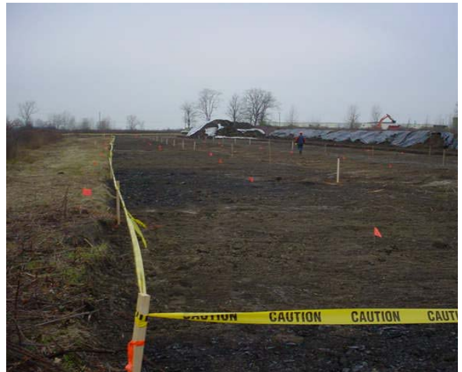
4.) AREA 1 – EXCAVATION, VIEWING NORTHWEST, STOCKPILED SOILS COVERED WITH POLYETHYLENE SHEETING IN BACKGROUND
