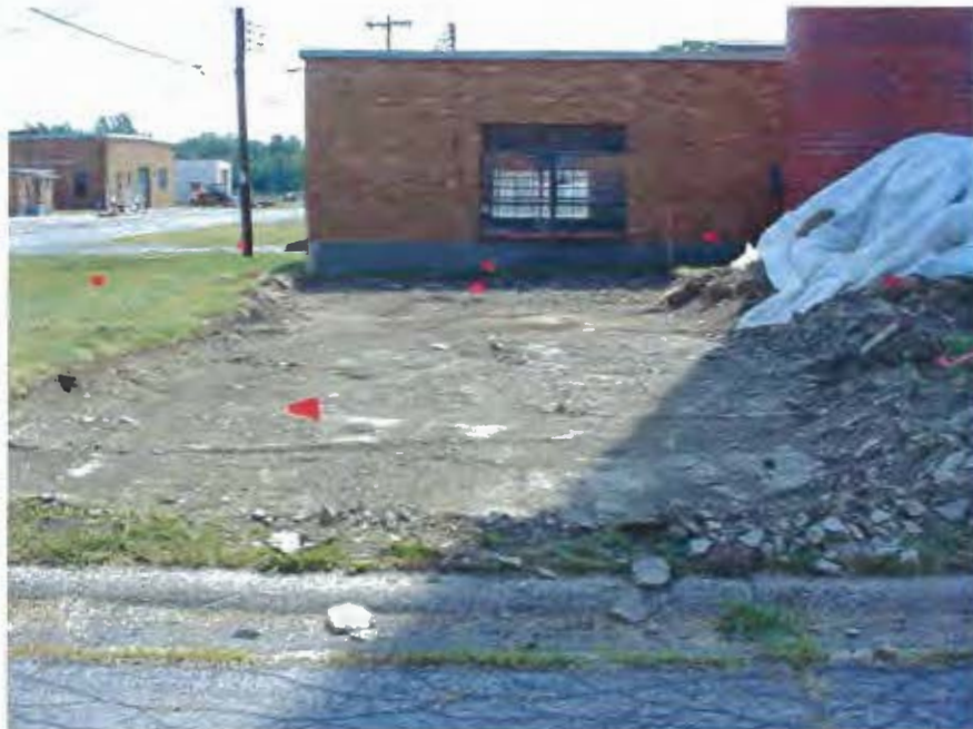
Photograph #2– View of the excavation area and post-excavation sample locations, marked with red flags at SEAD 39.
