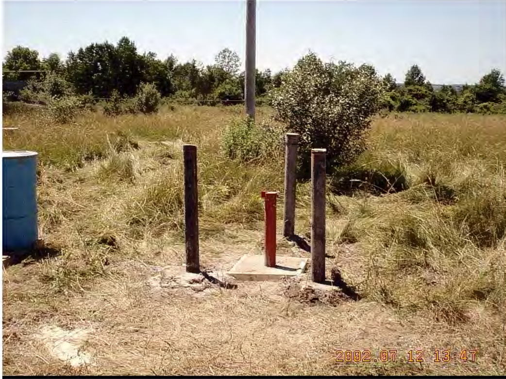
Status as of: 7/9/02 Description: View of monitoring well MW-3 after installation completed. Photo by: EJA
