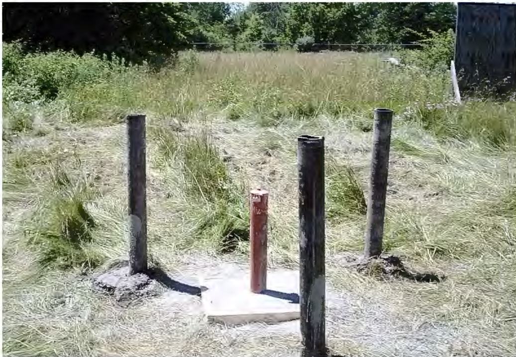
Status as of: 7/9/02 Description: View of monitoring well MW-2 after installation completed. Photo by: EJA
