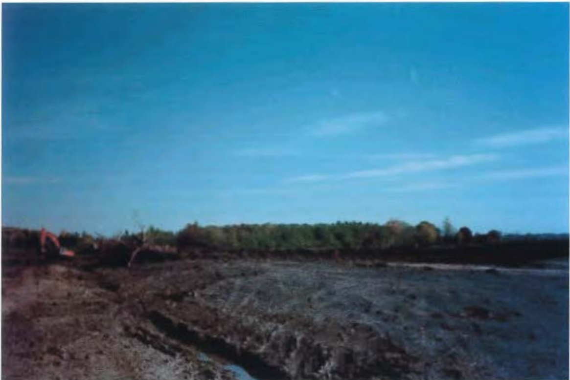
Figure G-12 Subcontractor draining rainwater from 44A.
