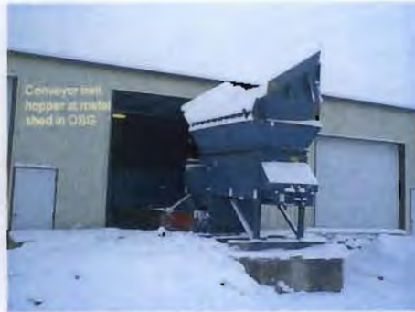
14. Conveyor hopper for metal to be Separated
