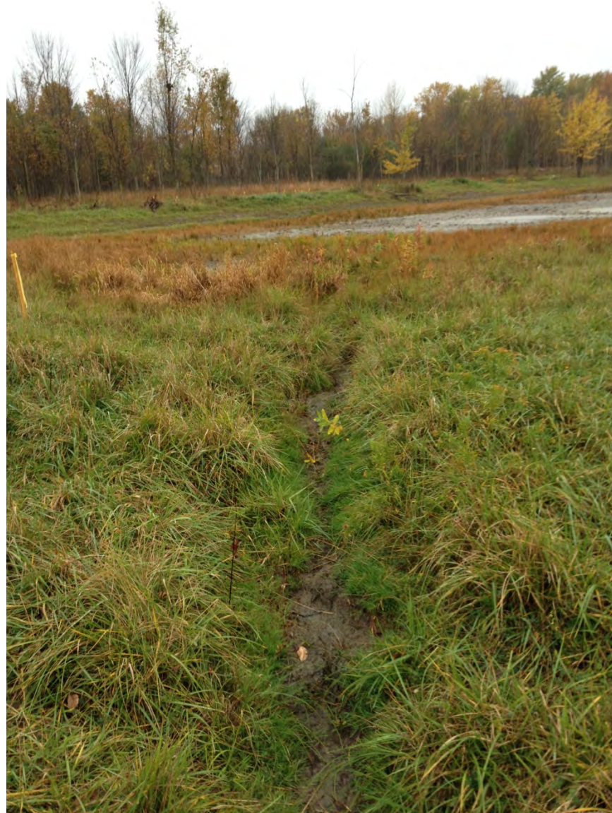
Photo #07 – Grid L8. No erosion or disturbances observed. Drainage ditch operating as intended. Well vegetated. Standing water across the road. View to the southwest.
