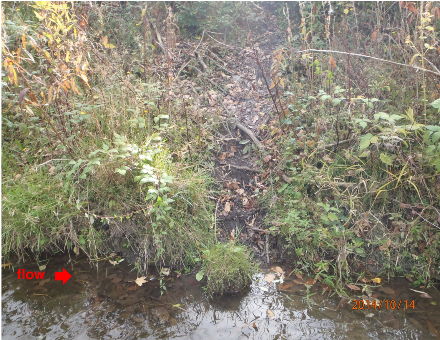
Photo #26 – Looking west at the creek embankment on OB grounds side of Reeder Creek. Vegetation and organics visible along the creek bottom.
