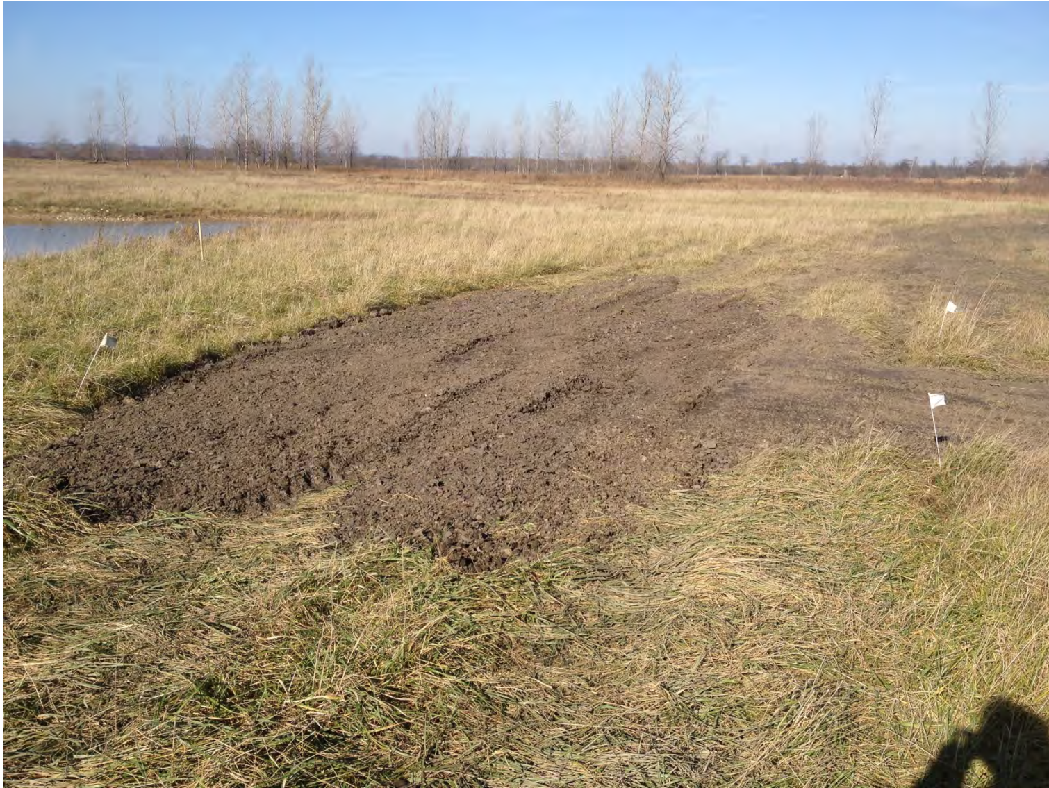
Photo #03b – Grid C7. Tire ruts were filled with a thin layer of crushed shale. The crushed shale was smoothed and graded without disturbing the underlying soil cap. View to the north.
