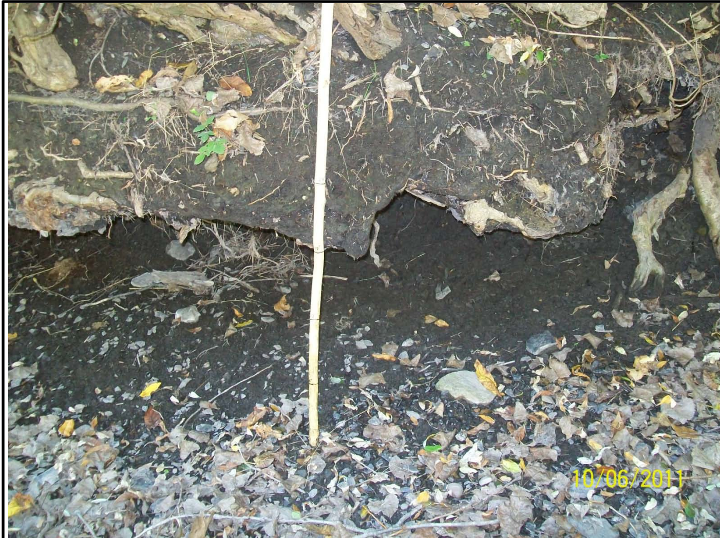
Photo #04 - Looking at west embankment (OB/OD Side) of Reeder Creek. Approximately 18 inches of creek bank have been scoured out beneath a tree located on the embankment; first observed in April 2009 inspection.
