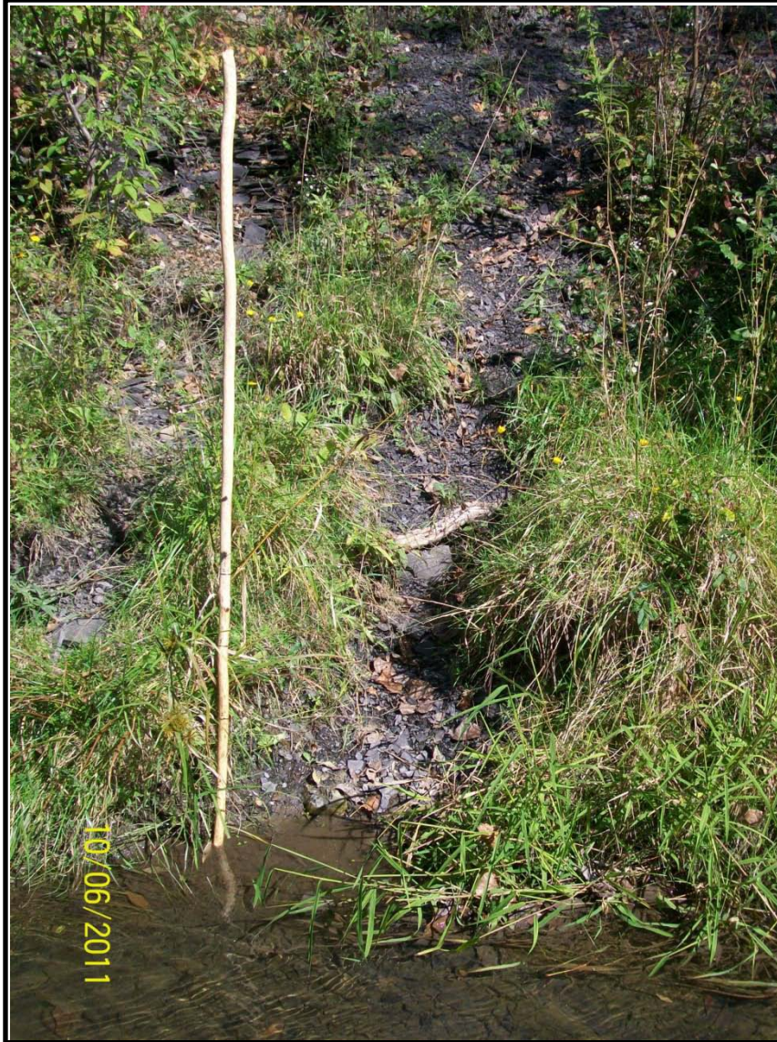
Photo #14 – Looking at east (SEAD-12) embankment of Reeder Creek. Embankment composed of shale layers with thin vegetated layer. Deer trails to creek are visible in photo.
