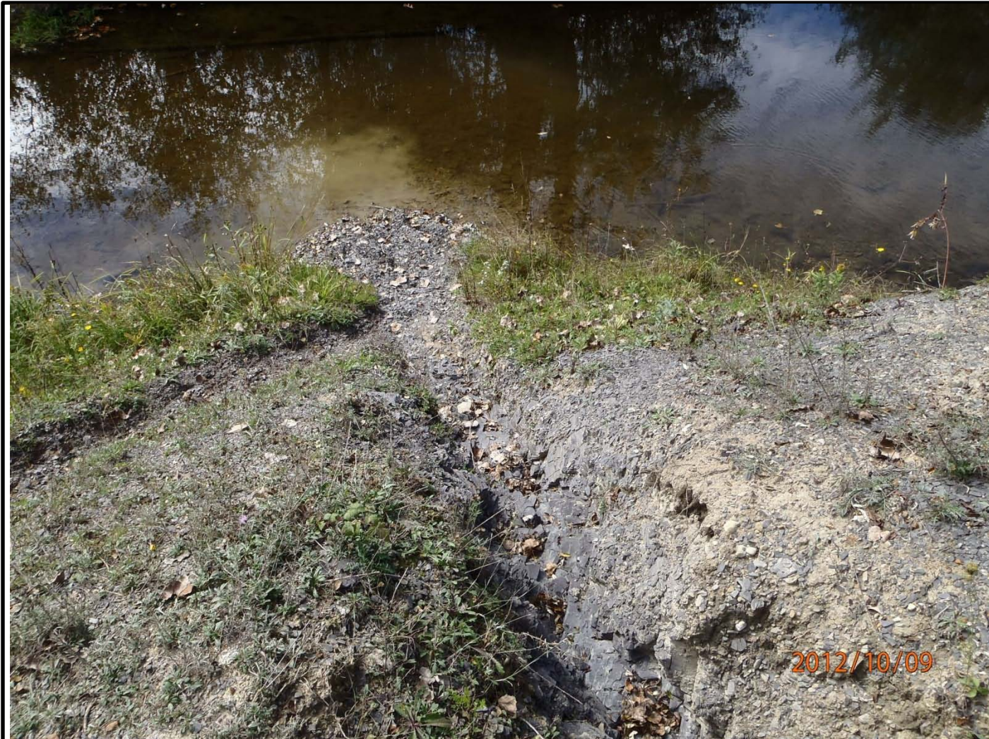
Photo #30 – Looking from on top of the east (SEAD-12) embankment of Reeder Creek. Embankment composed of shale layers with thin vegetated layer. Deer trails to creek are visible in photo. Deer trails cut into embankment 6-10 inches.
