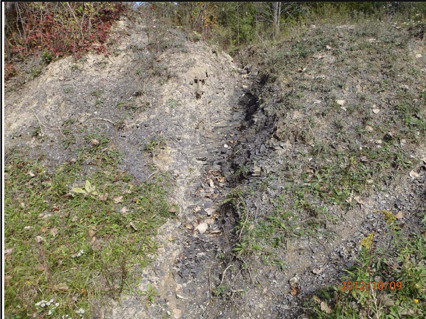
Photo #29 – Looking at east (SEAD-12) embankment of Reeder Creek. Embankment composed of shale layers with thin vegetated layer. Deer trails to creek are visible in photo. Deer trails cut into embankment 6-10 inches.
