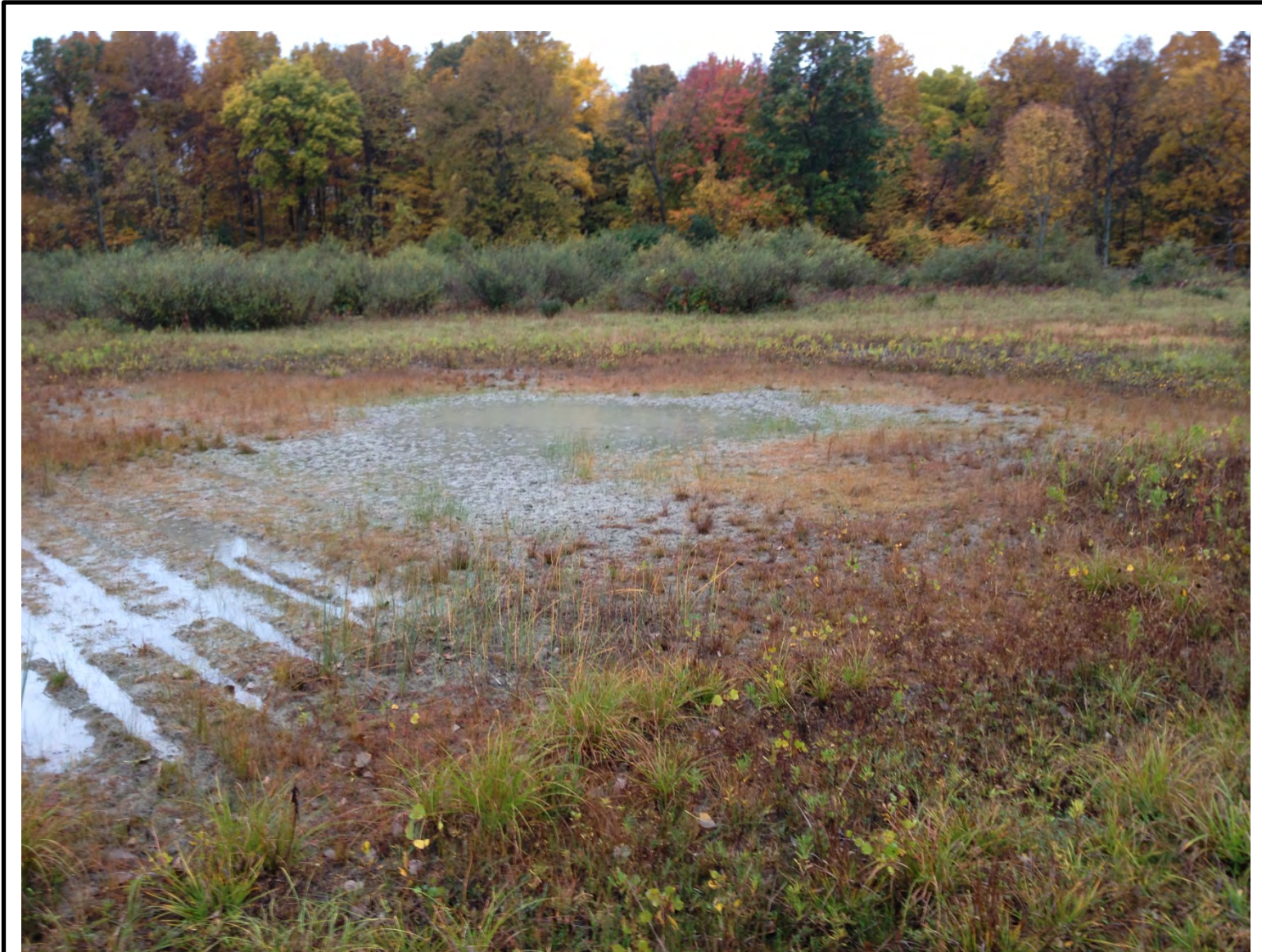
Photo #10 – Grid S8. No erosion observed in the cap areas. Ponding and shallow tire ruts are outside the area covered by the cap. Vegetated area in bottom right corner and right side of photo are limits of cap. View to the southwest.
