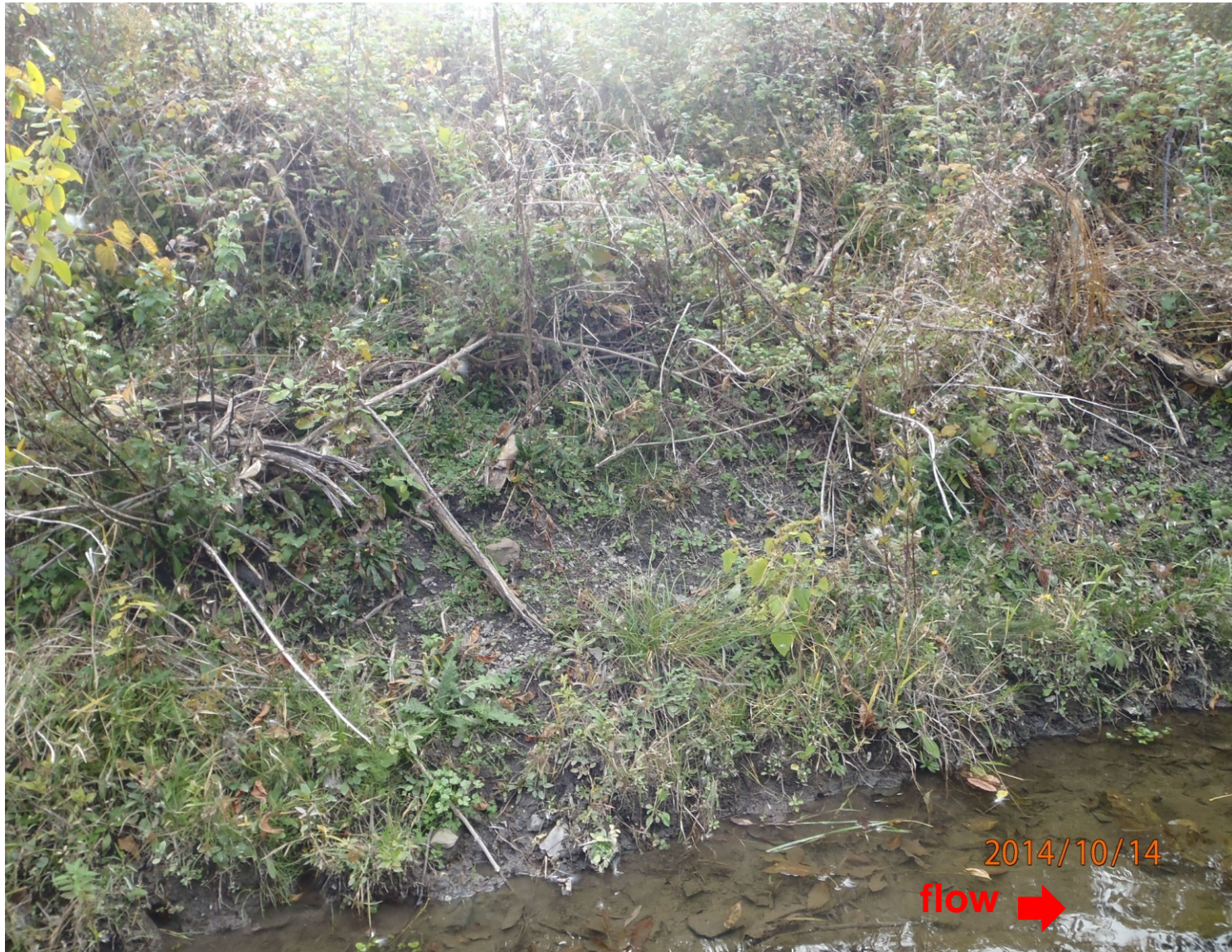
Photo #22 – Looking southwest at the creek embankment on the same side as the OB grounds. Creek embankment is very well vegetated and no evidence of overland soil transport exists.
