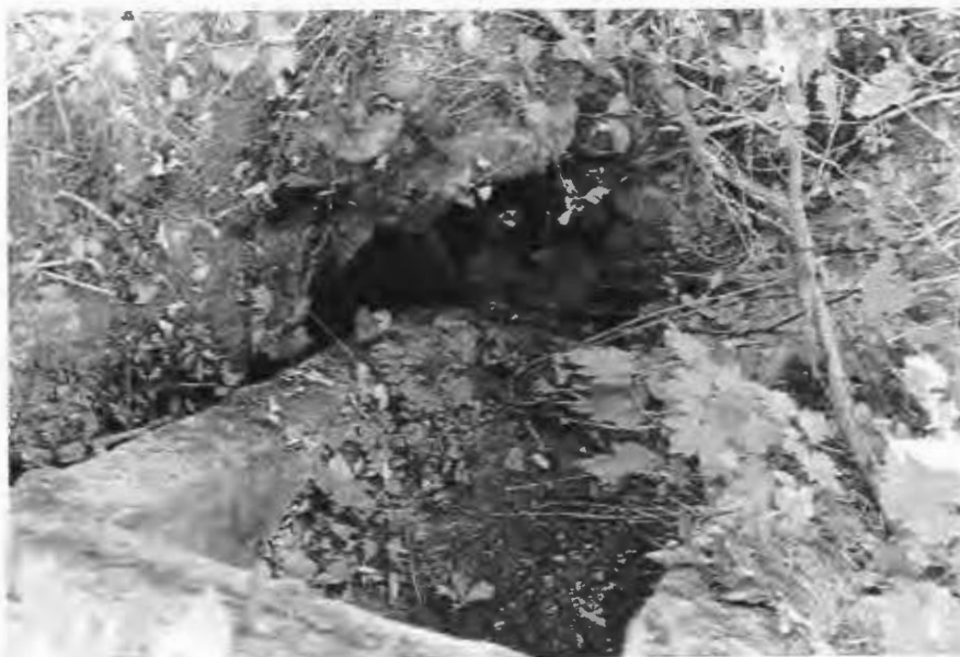
Figure 222. View of the rock-lined well with the cement trough pushed into it.
