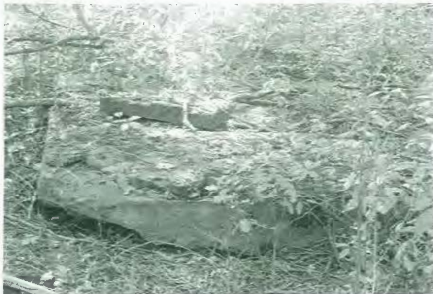
Figure 84. View of the displaced cement well cover at site A09906.000200.
