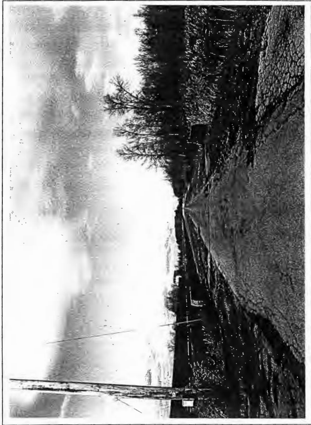
Figure 5-20. Culvert at West Patrol Road north of Indian Creek Road, facing north. Seneca Army Depot Activities, Seneca County, NY.
