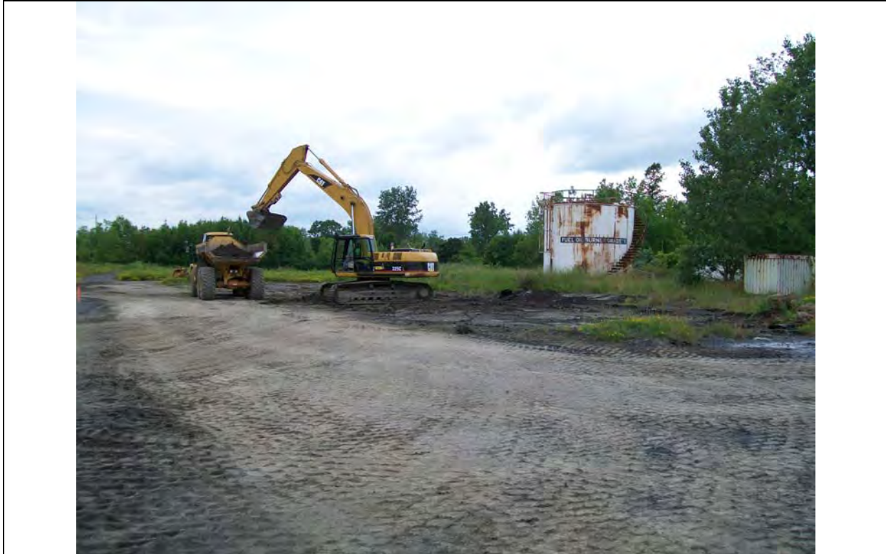
Photo: 11 Date: 7/7/2009 Site: SEAD-59 Description: Excavator nearly finished removing the SEAD-59/71 Additional Staging stockpiles.
