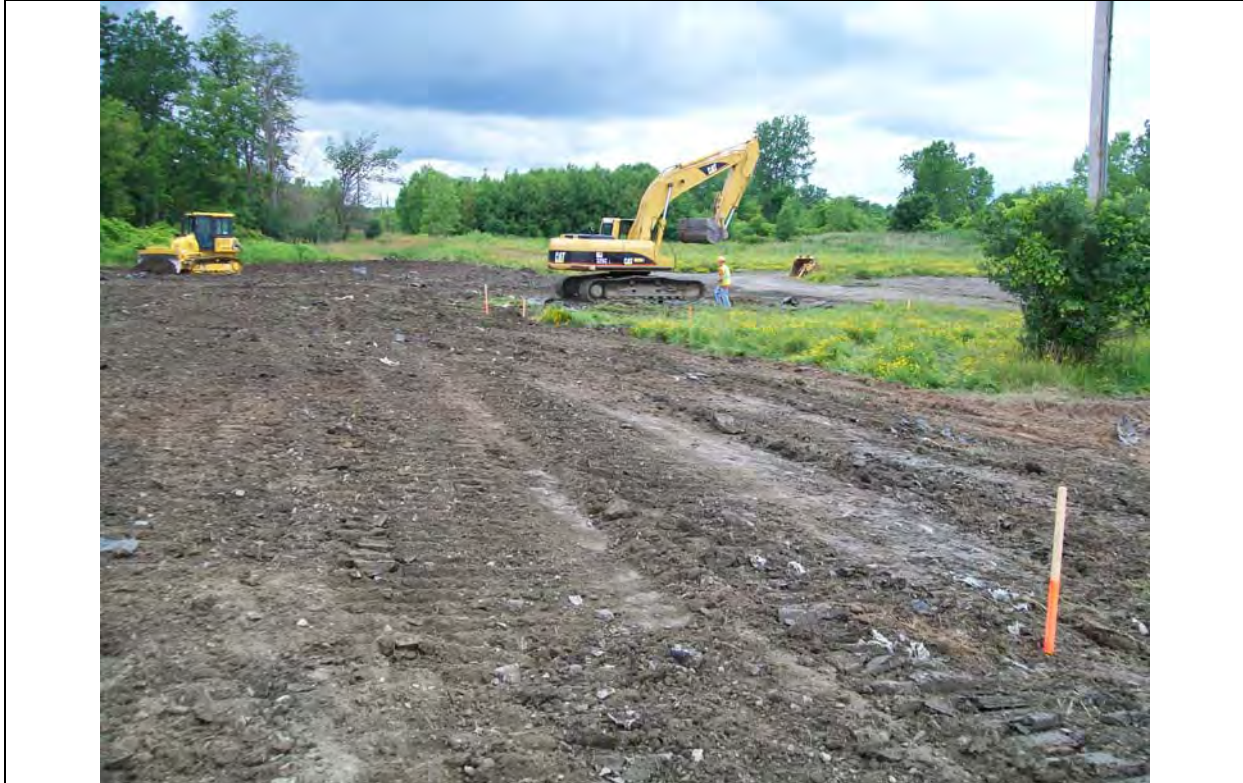
Photo: 12 Date: 7/8/2009 Site: SEAD-5 Description: Excavator running North-South across surface to compact of SEAD-59/71 stockpile soil cap.
