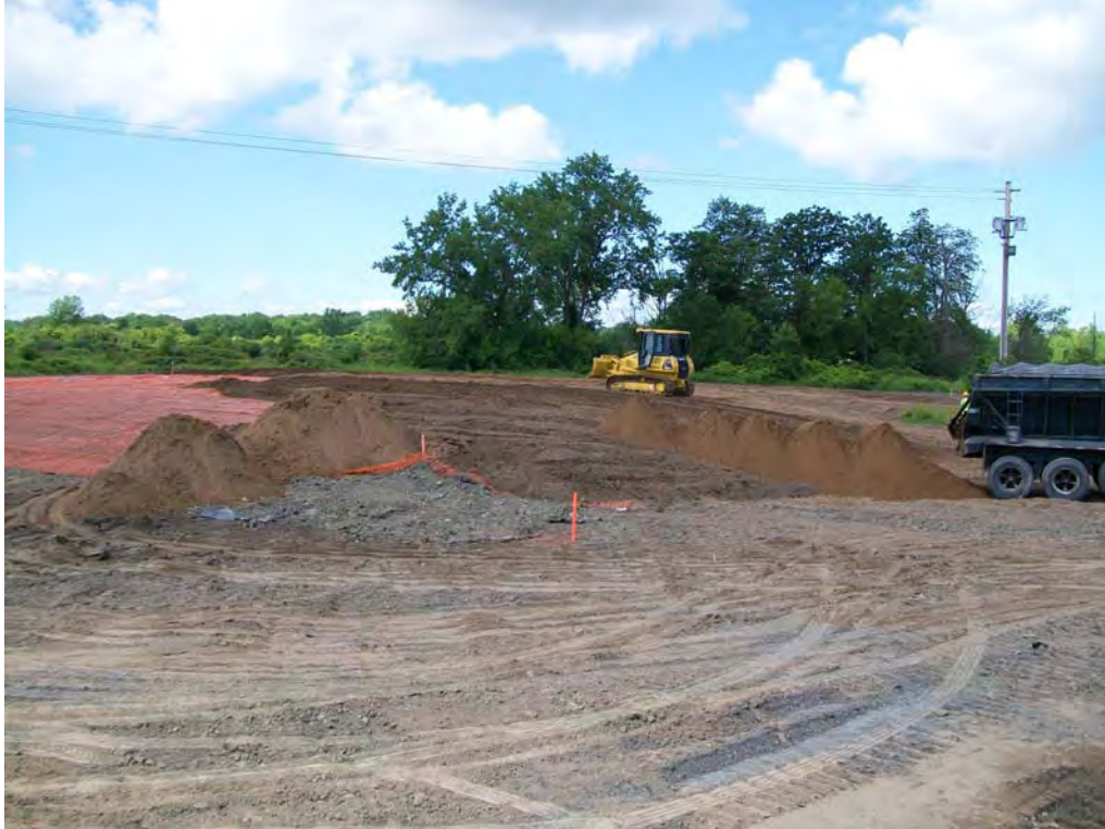
Photo: 17 Date: 7/9/2009 Site: SEAD-5 Description: Feathered edge of soil cap stake (solid orange) and top of soil cap final grade (stripe orange) in the Grid B-9.
