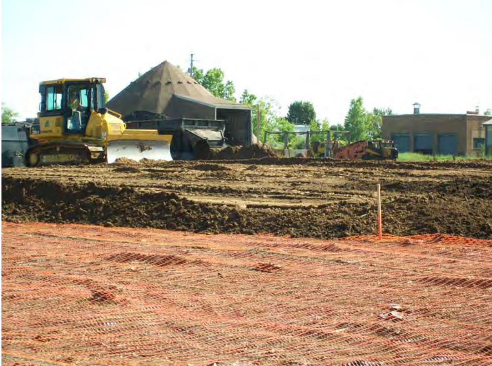
Photo: 16 Date: 7/9/2009 Site: SEAD-5 Description: Off-site borrow source material spread out to 1 foot thickness marked on the stake.
