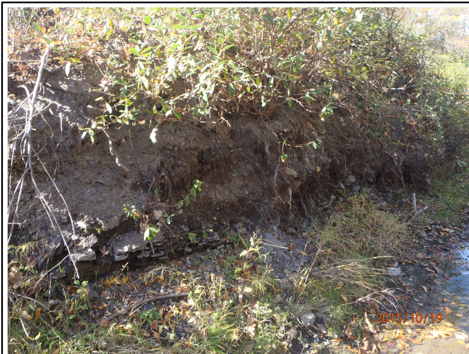
Photo #7 – Looking southwest at Reeder Creek’s western embankment. Considerable scouring on the embankment exposing soil from high flow event. Bottom of creek surface covered in fractured shale pieces and organics on top of bedrock.
