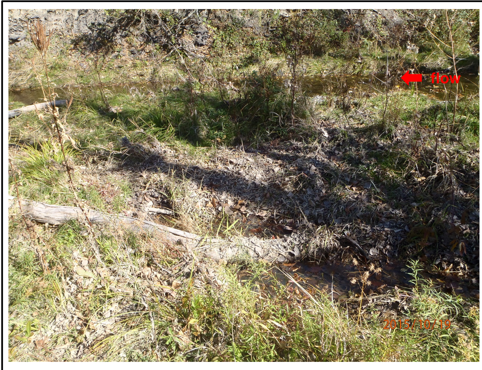
Photo #9 – Looking east at the flat, grassy embankment adjacent to Reeder Creek. Most of the vegetation was matted down and decomposing, indicating a high flow event through Reeder Creek. The low water level can be seen in the background flowing from right to left in this photo.
