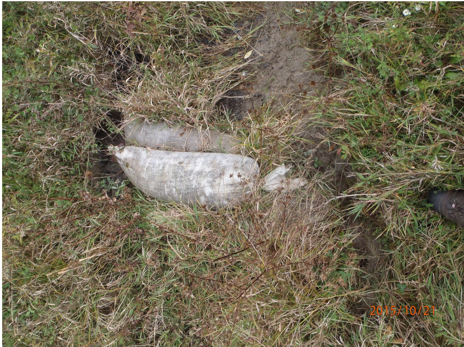
Photo #37 – View of sand bags in drainage ditch that leads down to Reeder Creek, located between MW23-1 and MW23-2. Flow through the drainage ditch during strong rain events has caused minor erosion around the perimeter of the sandbags. Erosion has created a new preferential flow path around the sand bags.
