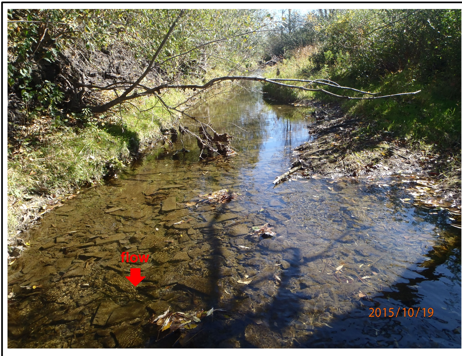
Photo #19 – Looking southeast (upstream) down Reeder. Fractured shale observed along the creek floor.
