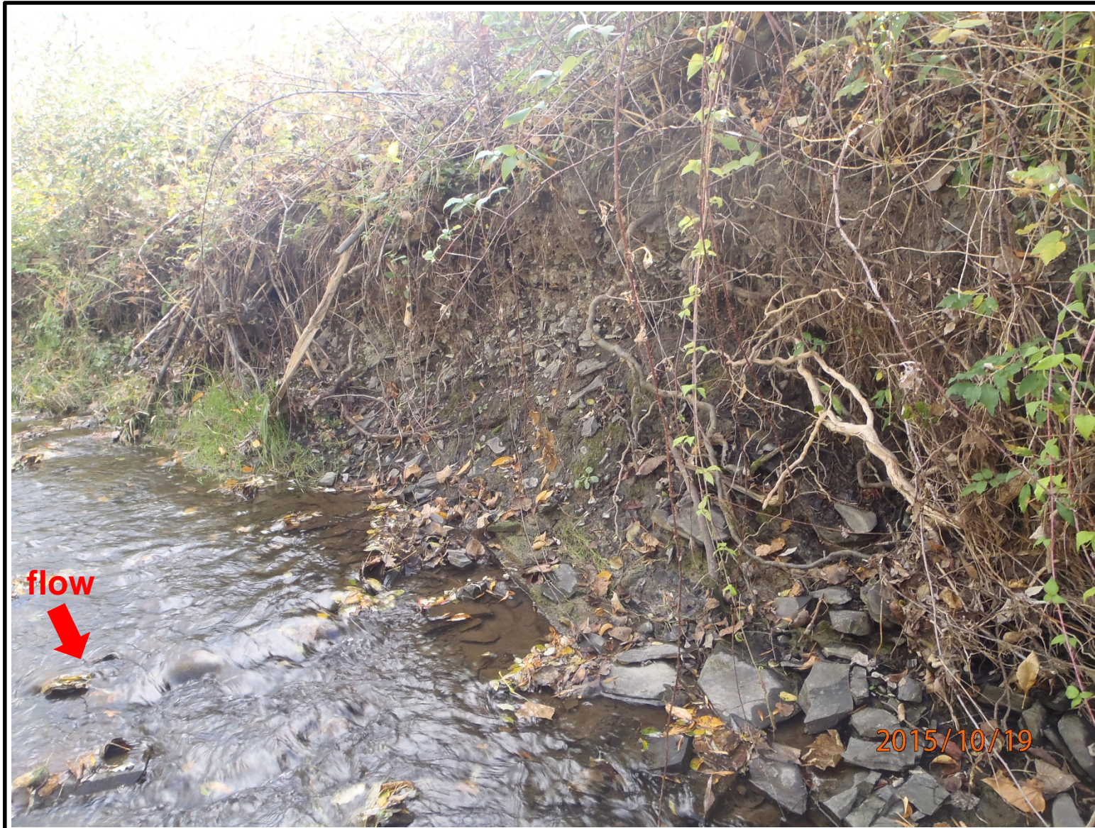
Photo #30 – Looking southwest at the steep embankment on the OB Grounds side of Reeder Creek. Visible soil within the embankment appears to show signs of scouring, likely during high flow event. No evidence of overland flow transporting soils from the OB Grounds to Reeder Creek.
