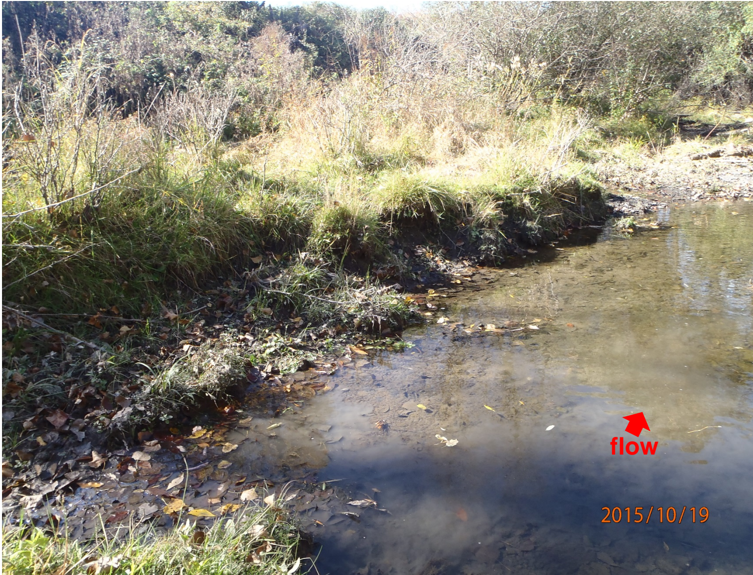
Photo #15 – Looking southwest at the western creek embankment (OB grounds side) of Reeder Creek. Local erosion of the embankment is present; however, no evidence present of overland flow occurring or excessive deposition of sediment into the creek. The embankment is densely vegetated.
