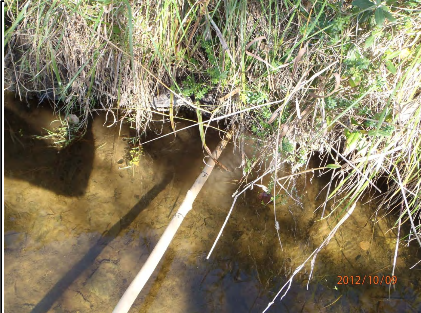
Photo #19 – Looking at west embankment (OB/OD Side) of Reeder Creek. Approximately 12 inches of creek bank have been scoured out along the embankment;.
