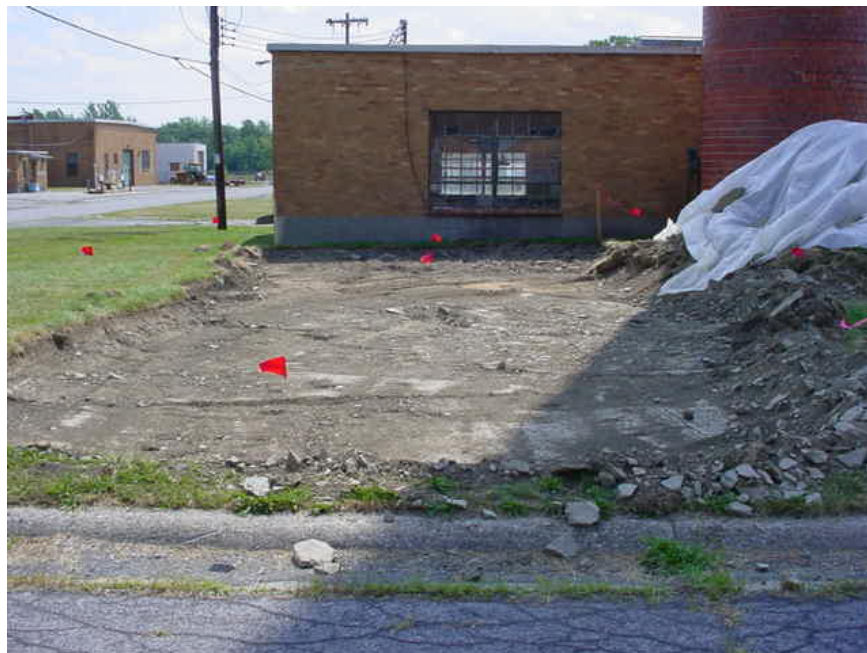
Photograph #2– View of the excavation area and post-excitation sample locations, marked with red flags at SEAD 39.
