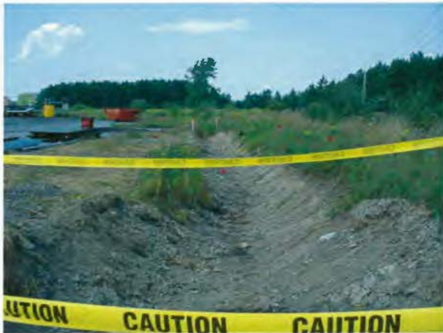
Photograph #6 – Caution tape was set up around the ditch with 6-ft excavation at SEAD 40.
