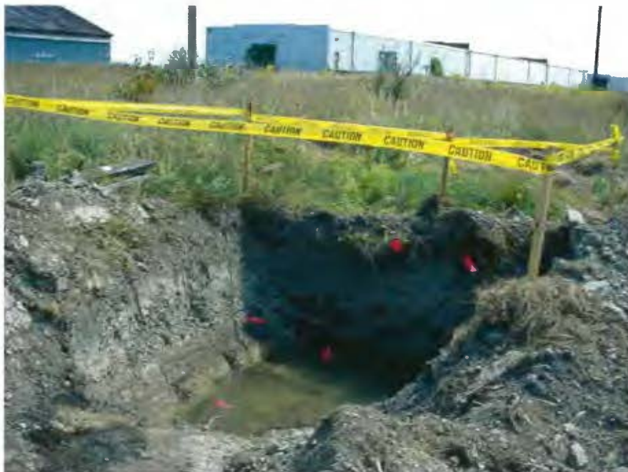
Photograph #4- View of the northern portion of the ditch with 6-ft excavation at SEAD 40.
