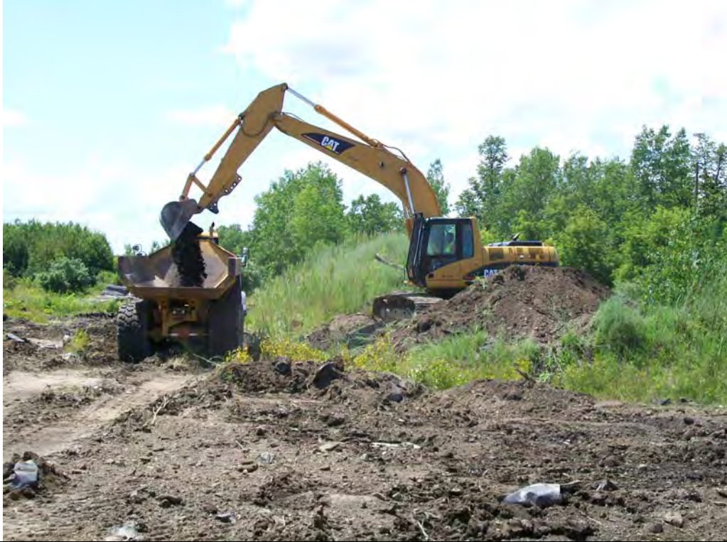
Photo: 7 Date: 7/6/2009 Site: SEAD-59 Description: Excavator loading haul truck with material from the SEAD-59/71 North Staging stockpiles.
