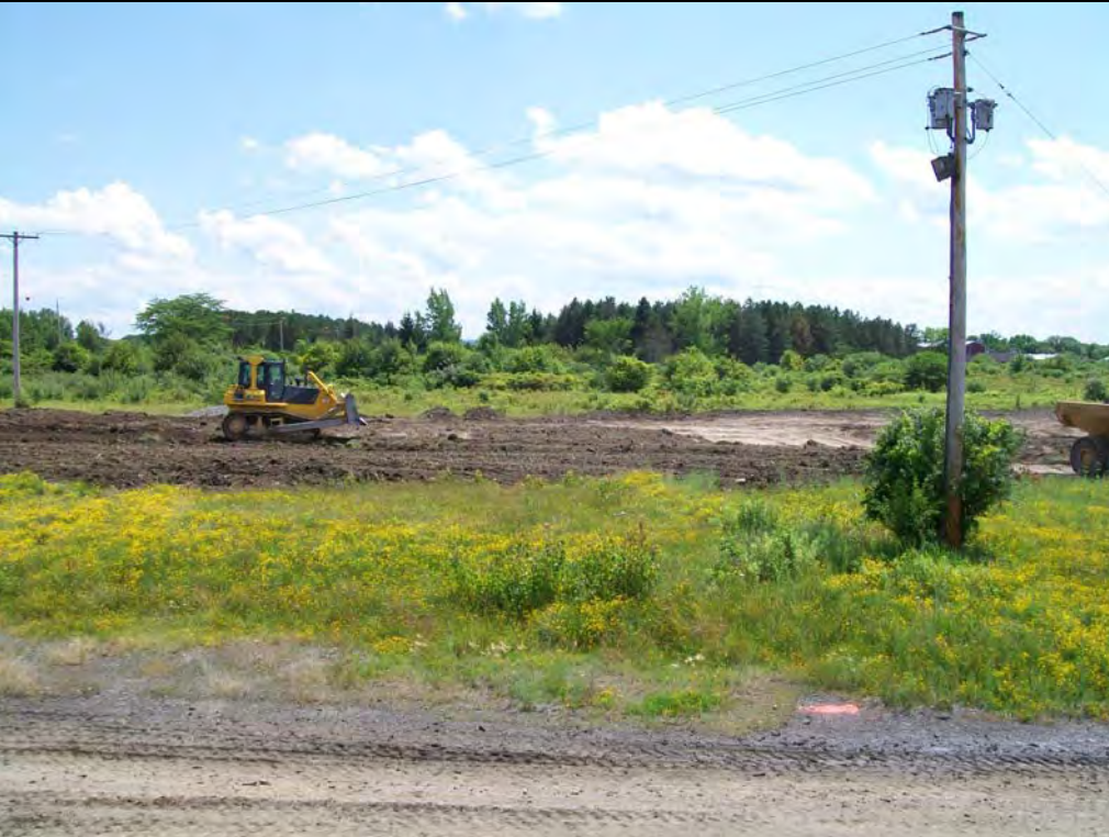
Photo: 6 Date: 7/6/2009 Site: SEAD-5 Description: Bull dozer spreading out SEAD-59/71 South Staging stockpile across the SEAD-5 soil cap limits.
