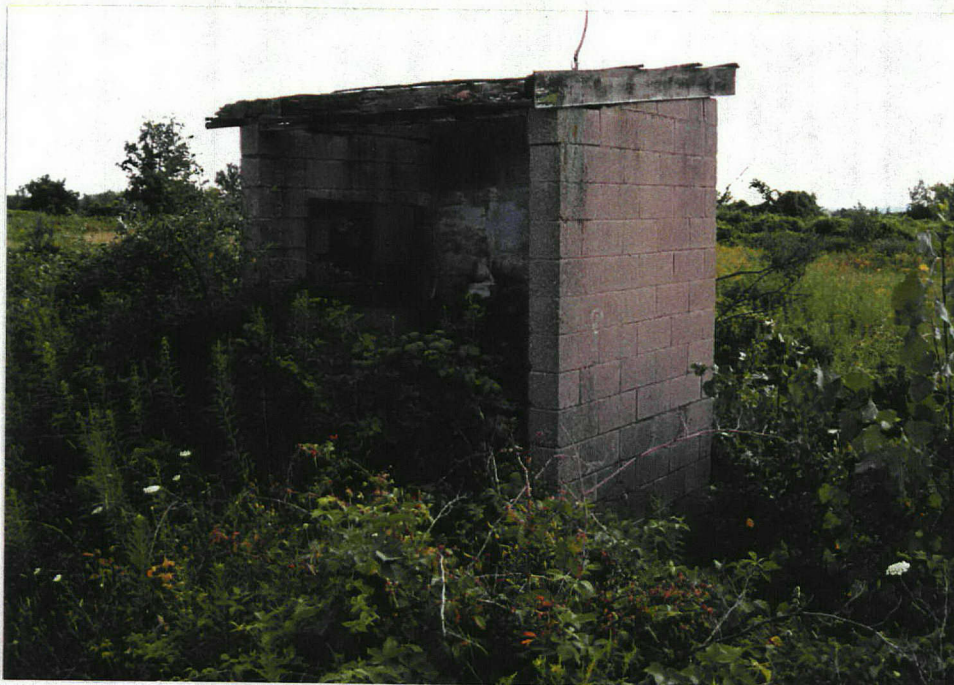
PHOTO # 39 DETONATOR DESTRUCTION FURNACE
