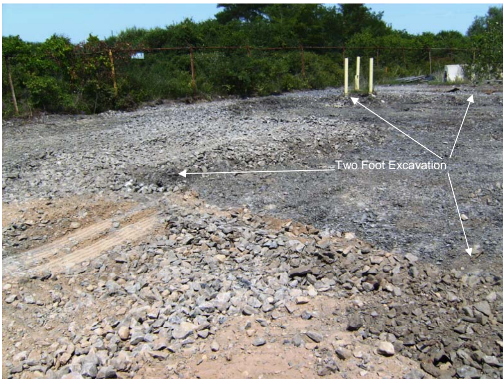
Two-Foot Excavation in Northeast Corner And in Vicinity of Monitoring Well MW121C-3 Looking North, Northwest
