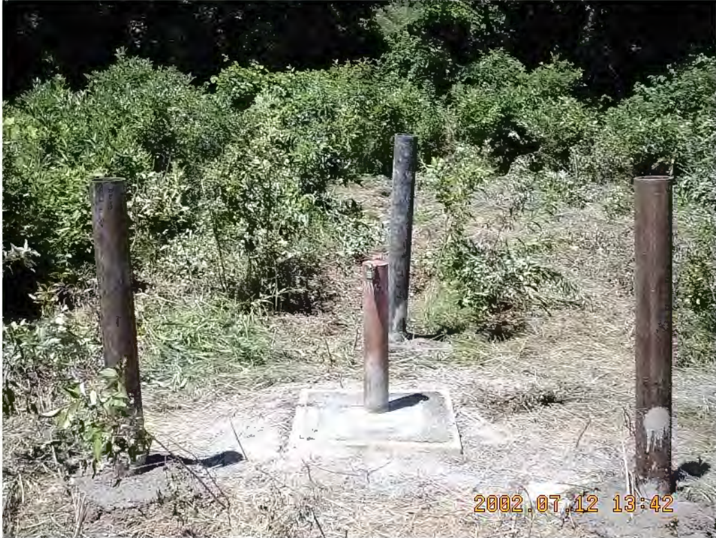
Status as of: 7/9/02 Description: View of monitoring well MW-1 after installation completed. Photo by: EJA
