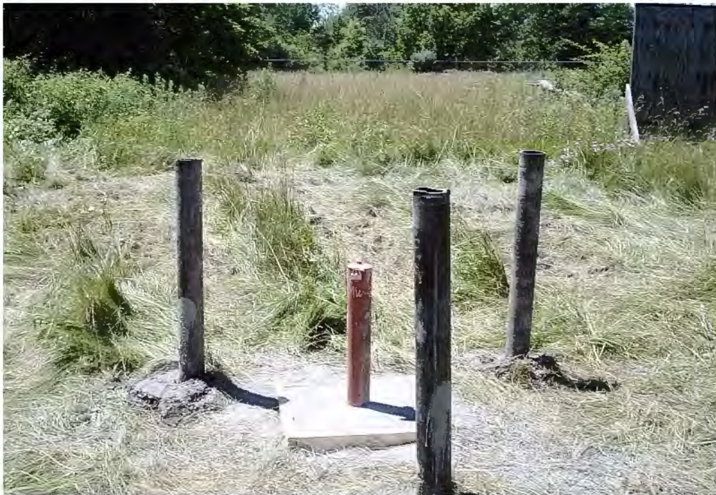
Status as of: 7/9/02 Description: View of monitoring well MW-2 after installation completed. Photo by: EJA
