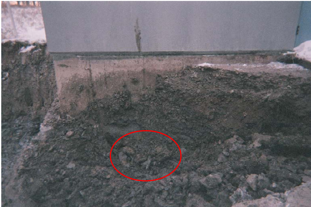
Remains of 4-inch Ductile Iron pipe
