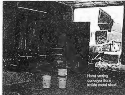
16. Hand sorting line inside metal shed w/safety shield
