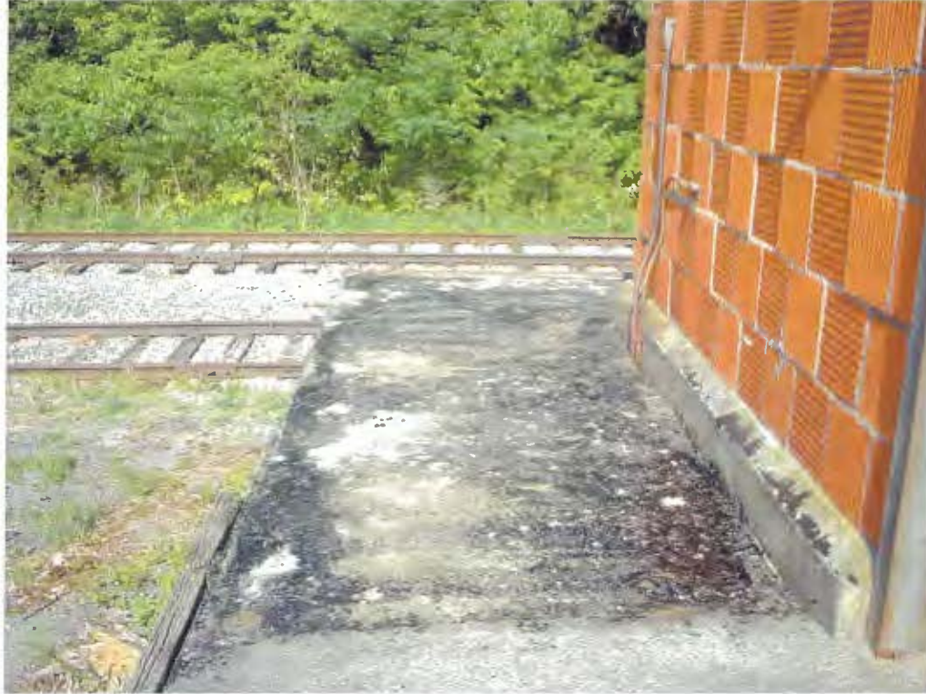
Figure 5: Northeast Corner of Building 301 (SEAD-2) Loading Dock with Asphalt/Gravel Traction covering removed.
