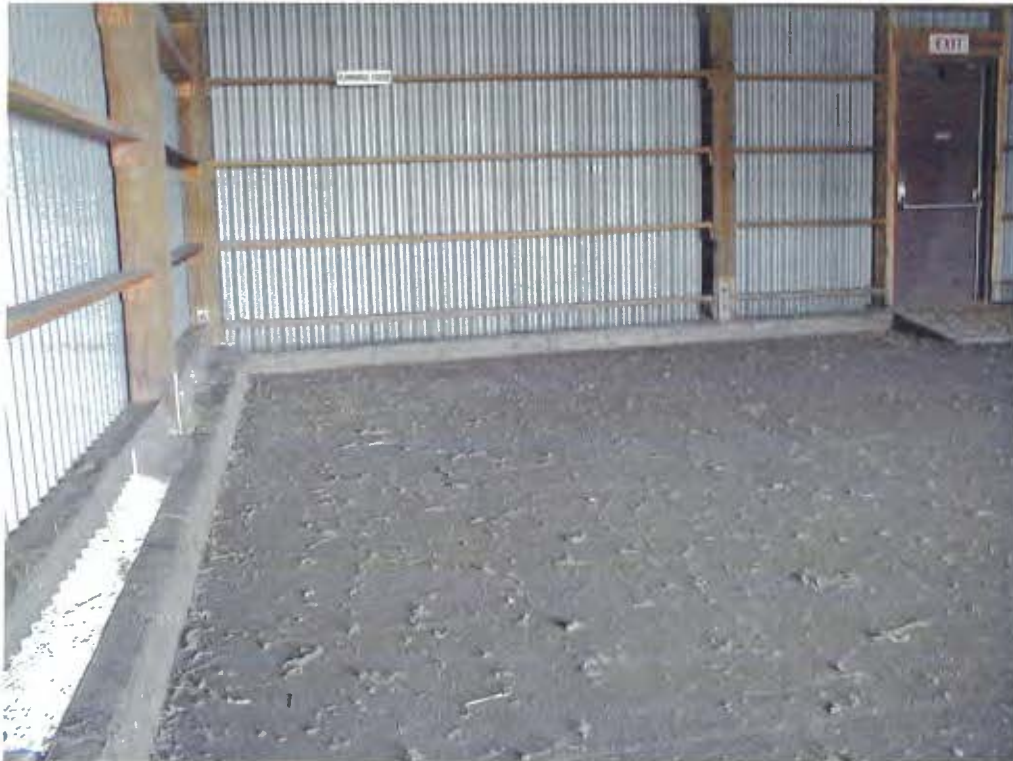
Figure 1: Interior of Building 307 (SEAD-1) prior to decontamination monolithic floor and berm, lower passive ventilation area and sheet metal walls.
