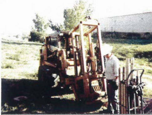
U.S. DoD and DOE representatives conduct a joint evaluation of the hydraulic performance of PRBs at former Lowry Air Force Base
