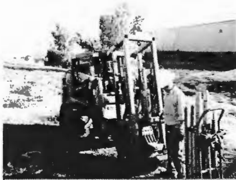
U.S. DoD and DOE representatives conduct a joint evaluation of the hydraulic performance of PRBs at former Lowry Air Force Base
